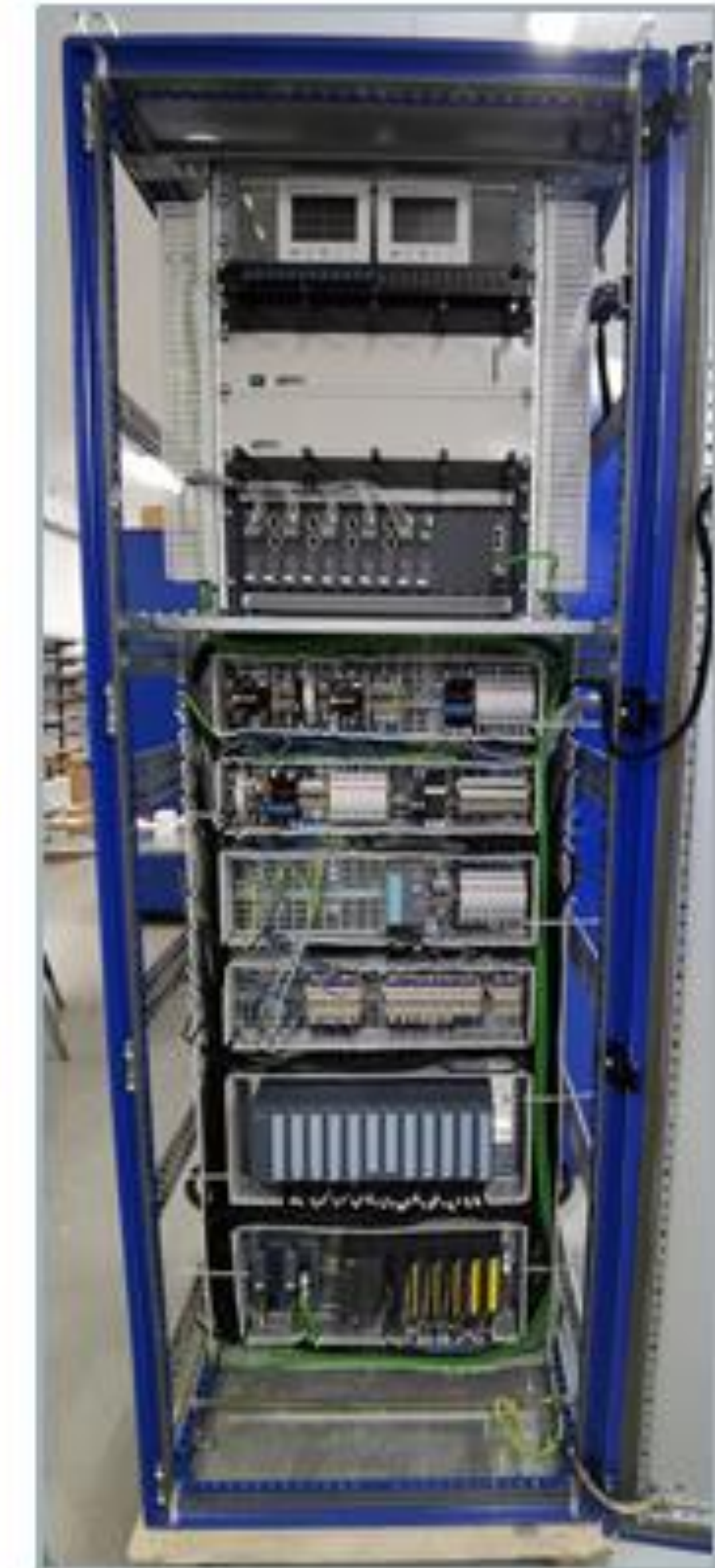
Cryopump Control Cubicle
