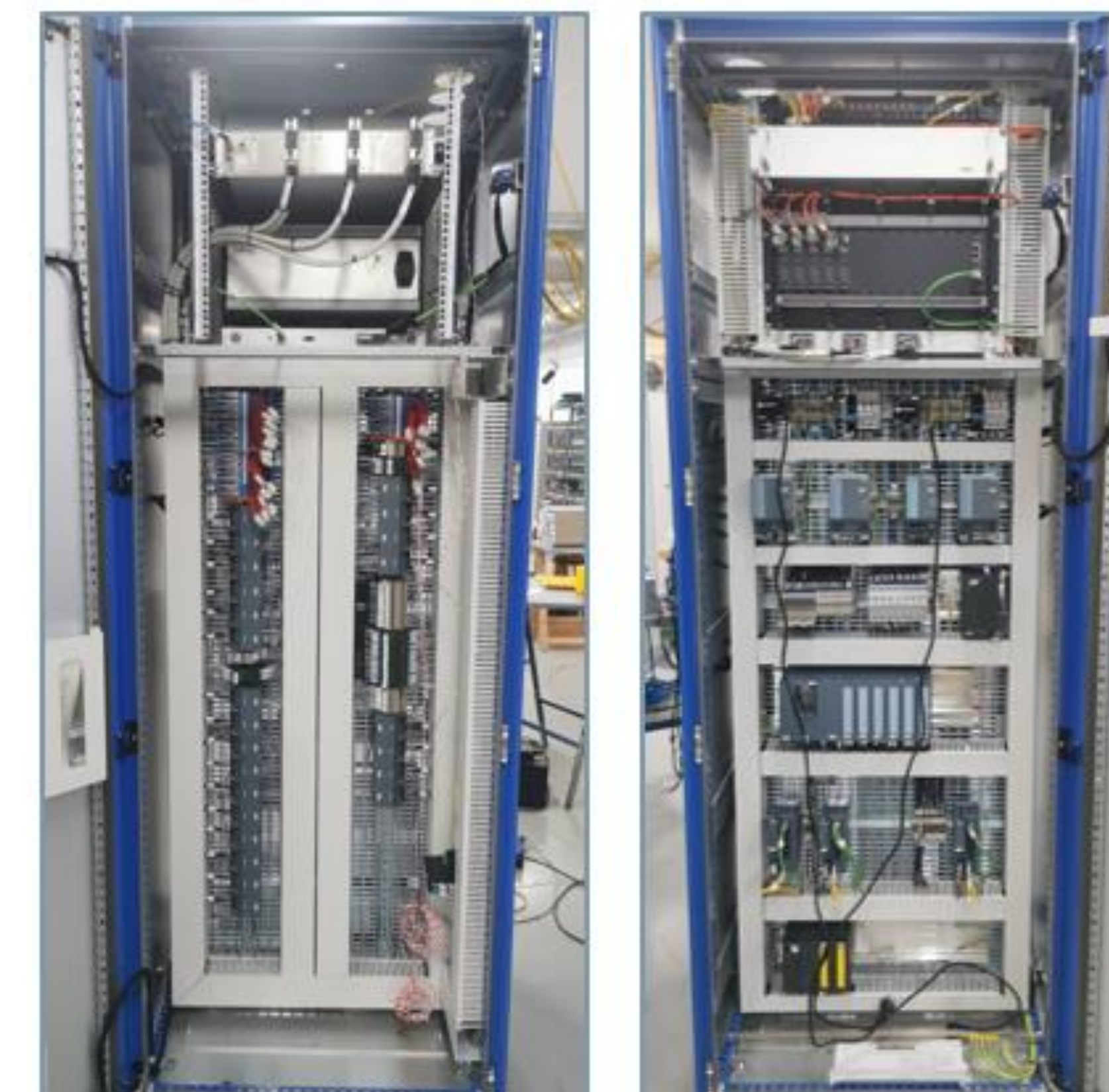
Warm Regeneration Box Control Cubicle
