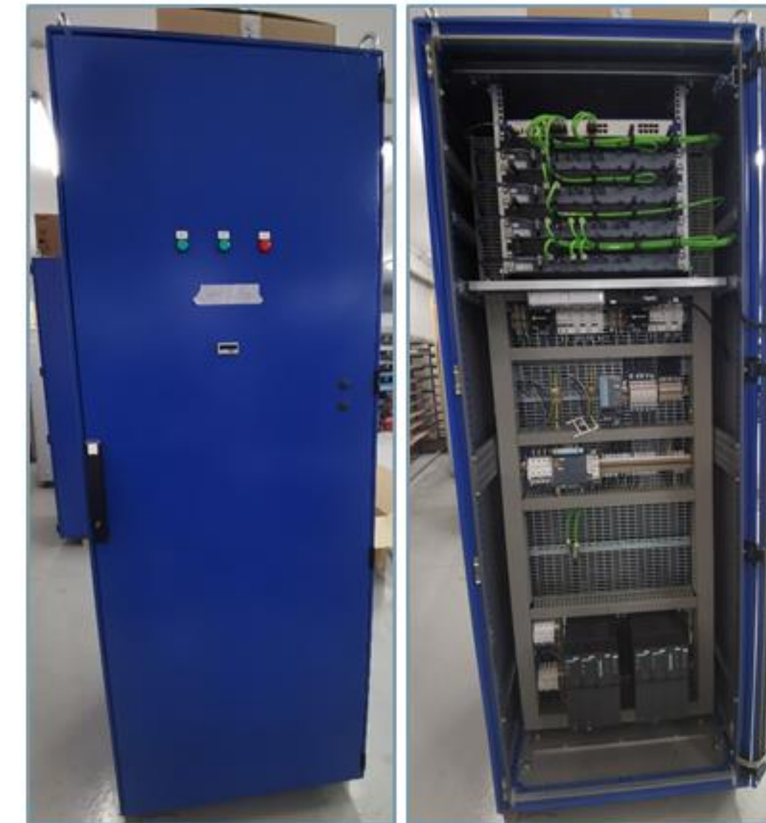
Master Control Cubicle
