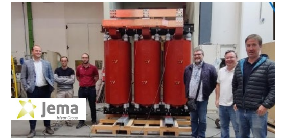
TFC PS ML/LV Transformer
